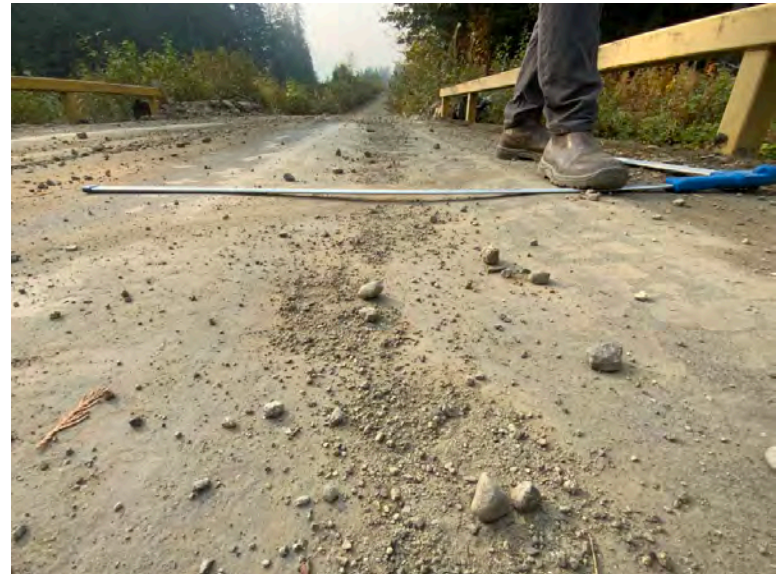
Deck buckle under wheel track upstream.
