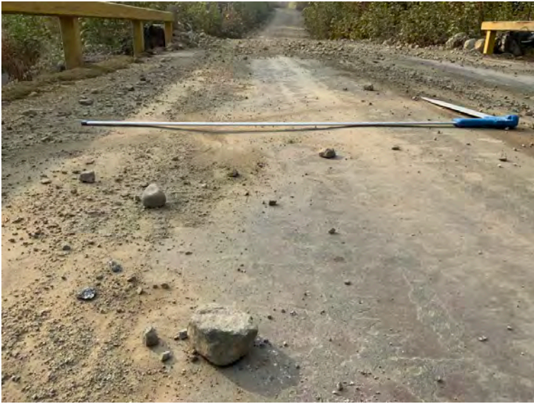
Deck buckle under wheel track downstream
